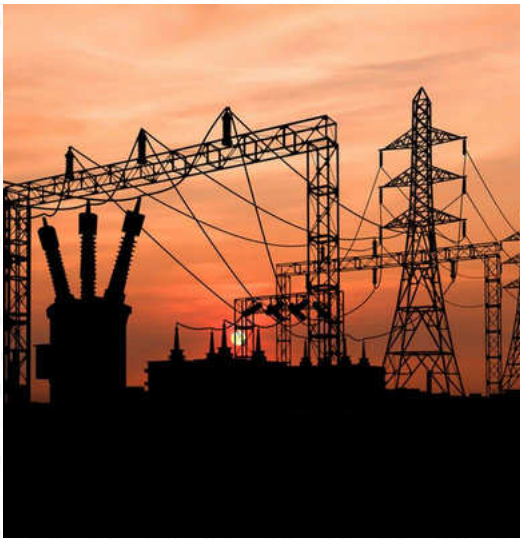
Reliable and Uninterrupted Industrial Utilities
